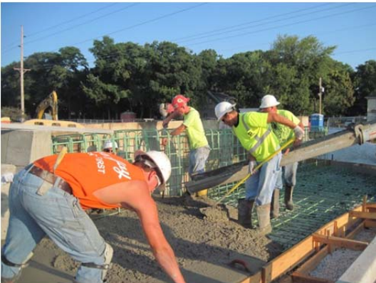
Photo 22: Workers pour anchor slab sidewalk off NW corner of Race Street Bridge.
