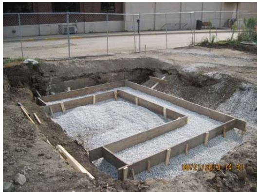
Photo 16: Foundation form for planter wall at NW corner of Griggs and Race Street.
